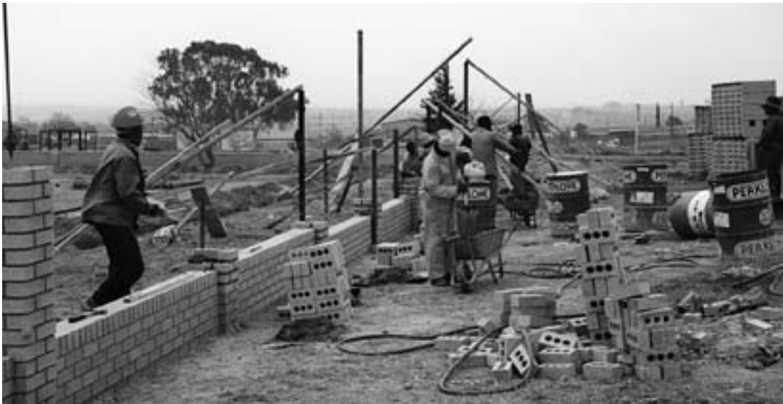
Emerging contractors benefiting from a loan from the Mpumalanga Economic Empowerment Corporation refurbish the local Magistrates' offices at Kwaggafontein.
